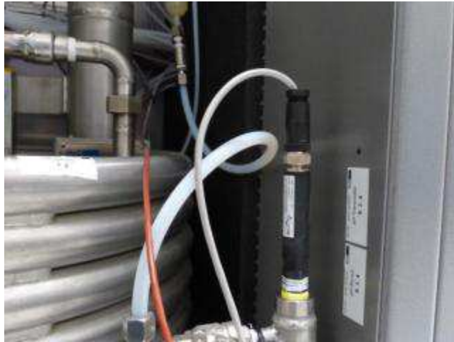
Fig.2-4: JUMO sensors for measuring pressure, conductivity, and pH in the vacuum distillation plant.
